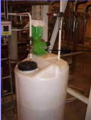
Chemical Metering pump
