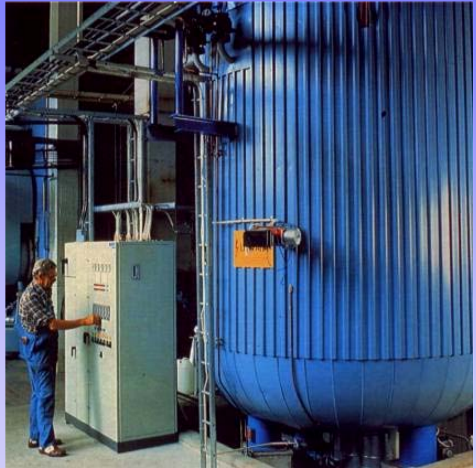
Astra, Sweden, 12MW, 6kV, 23 bar
